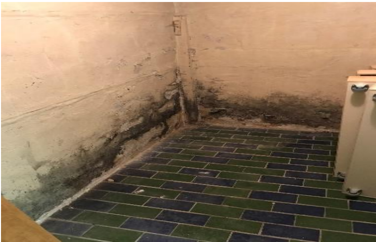
Photo 4: View of suspect mold growth observed on concrete walls in the basement of the subject building.
