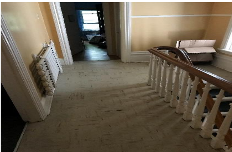
Photo 2: View of asbestos-containing vinyl floor tile observed in the 1 st floor landing.
