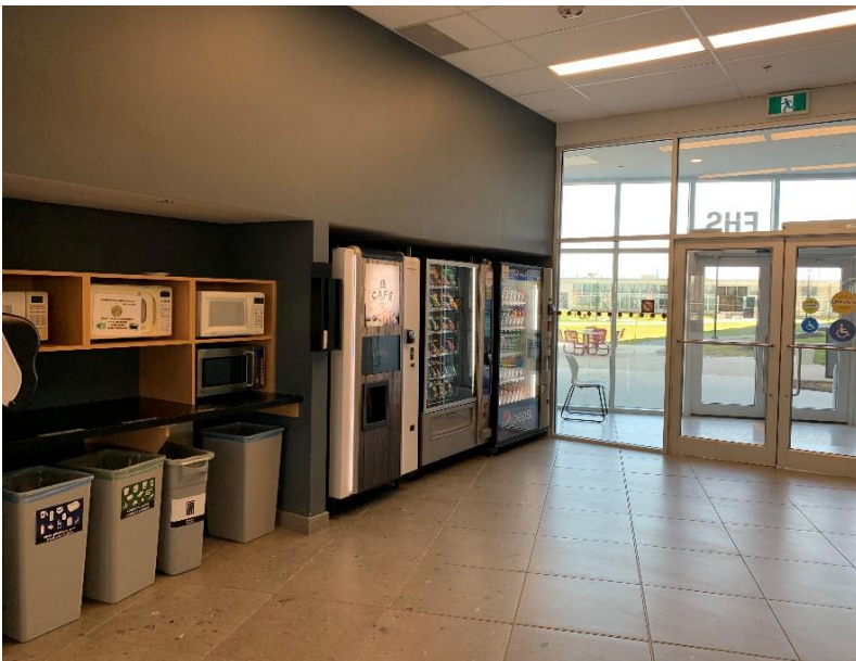
Photo 4: View of refrigerators containing ozone depleting substances.
