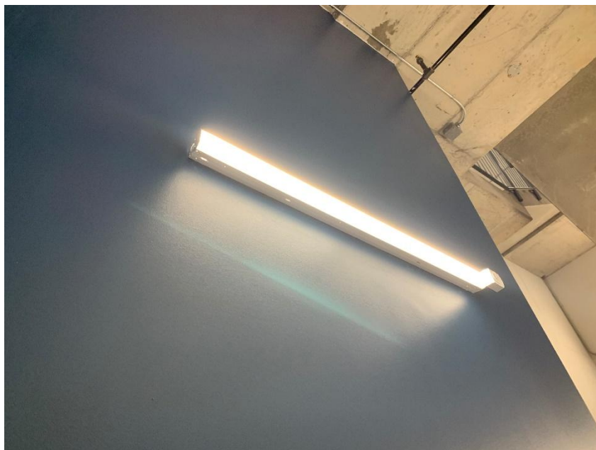
Photo 9: Lead-acid batteries present in emergency lights
