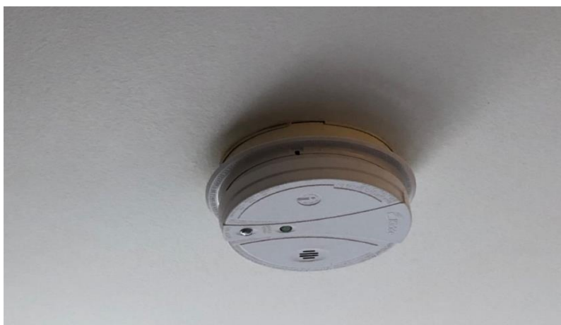
Photo 12: Typical view of smoke detectors containing radioactive materials.
